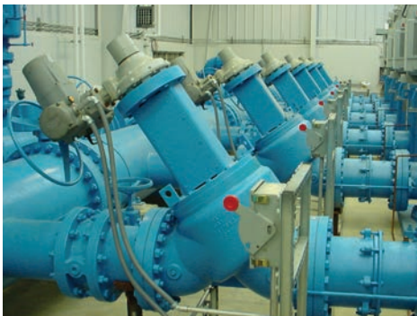
Olentangy Water Treatment Plant, Ohio, USA 6 – 14" CHECKtronic® Pump Control Valves
