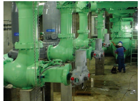
DELCO Raw Water Pump Station, Ohio, USA 3 – 14" Checktronic® Pump Control Valves
