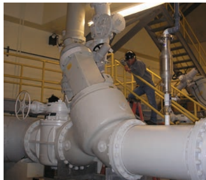
Brooks Road Sewage Pump Station, Georgia, USA 2 – 24" Checktronic® Pump Control Valves
